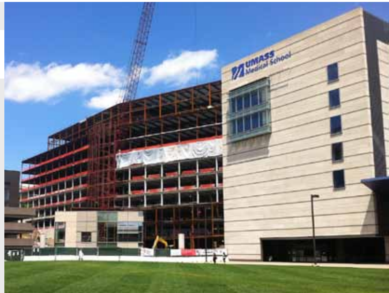
Currently under construction—the University of Massachusetts Medical School Albert Sherman Center in Worcester, Massachusetts. Photo courtesy of Fore Solutions.
