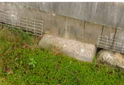
Above top: Interior dining room window. Above bottom: Shingle wall base. The foundation, which really was pretty good... considering. Very well drained soil kept it from collapsing. Photos courtesy of Knight Associates.
