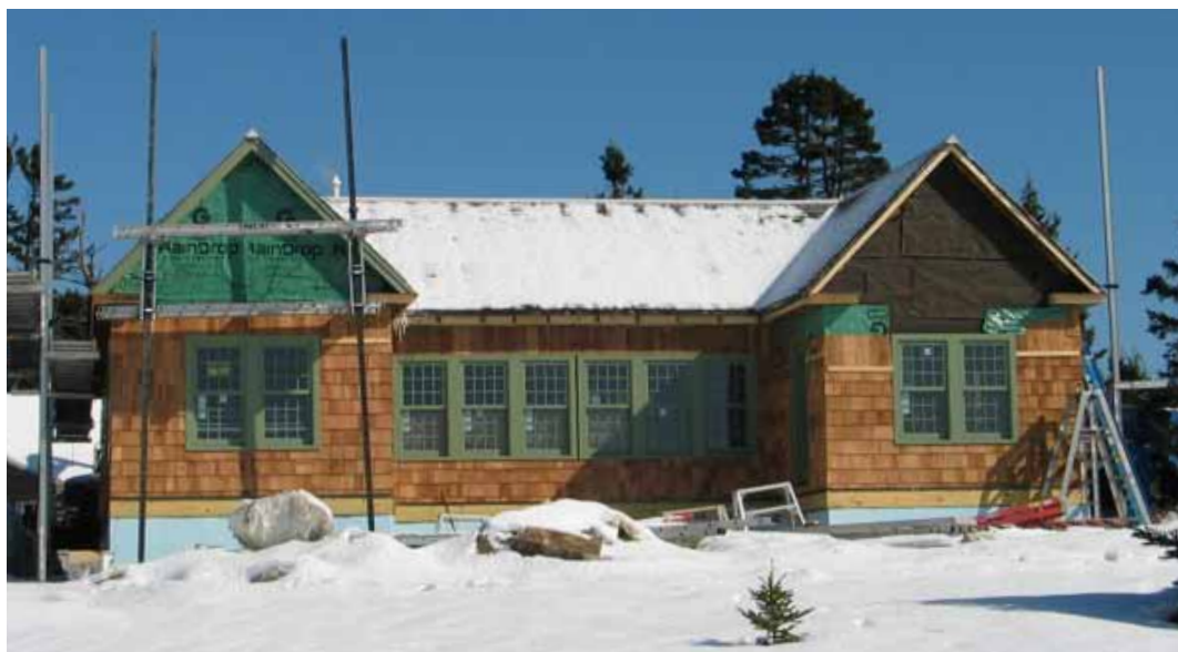
Above top: House on cribbing. We moved it, built a foundation under where it had been, and moved it back. Project architect Richard Manzo and I felt it important that it stay exactly where it was. Now, Windswept is much stronger. We reinforced most of the truly daring framing (2 x 4 rafters on 30" centers). It has been on an insanely exposed site for almost 100 years and was pretty straight. Maybe we don't need that code! Above bottom: House in snow with green windows. The color change on the outside comes from the book, which talked about dark green trim, but also talked about colors to match the sea outside. We opted for a muted green, and our new shingles will soon be gray. Photos courtesy of Knight Associates.
